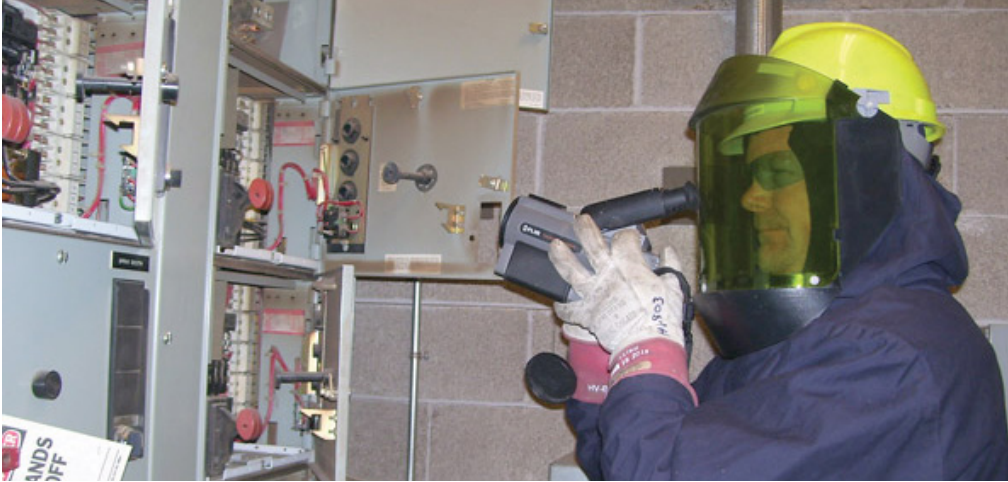
Figure 5 Infrared Scanning is applicable on all electrical assets including Motor Control Centers but typically requires extensive PPE if done “open panel”
