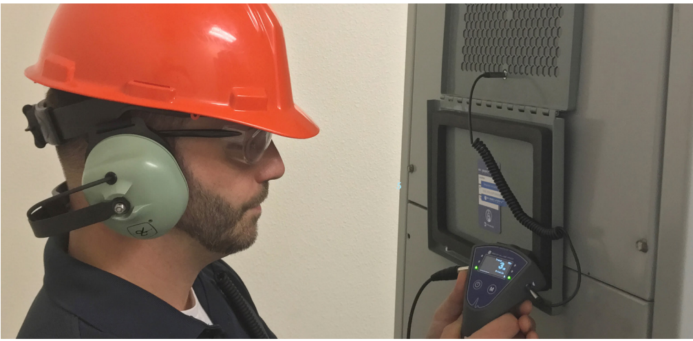
Figure 7 An IRISS Maintenance Inspection window for visual, Infrared, Ultraviolet and Ultrasound inspections installed on medium voltage switchgear; no special PPE is required to use the EMSD
