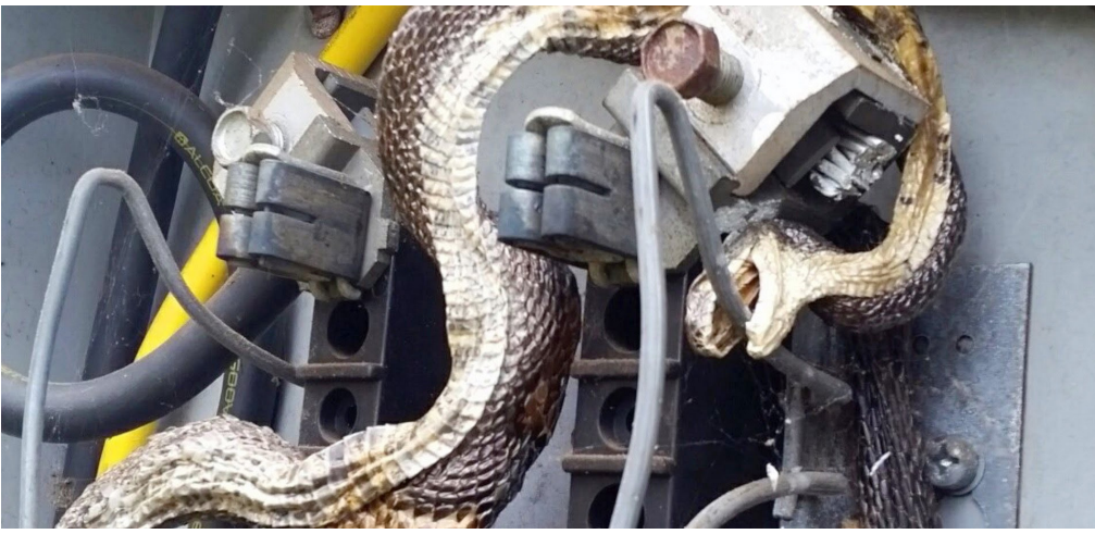
Figure 3 Pests and their predators can be attracted to warm, dry spaces inside transformers
