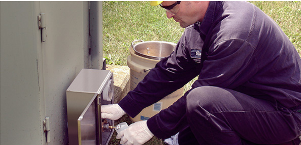
Figure 8 A safer oil sampling method retrofitted to an existing transformer allows energized sample collection; the sampling cabinet is lockable to prevent unauthorized access. (Courtesy SDMyers)
