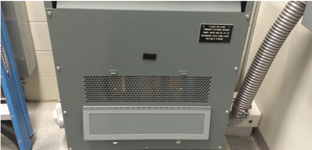
Figure 12 Custom replacement dry transformer panel-front with built in Maintenance Inspection Window
